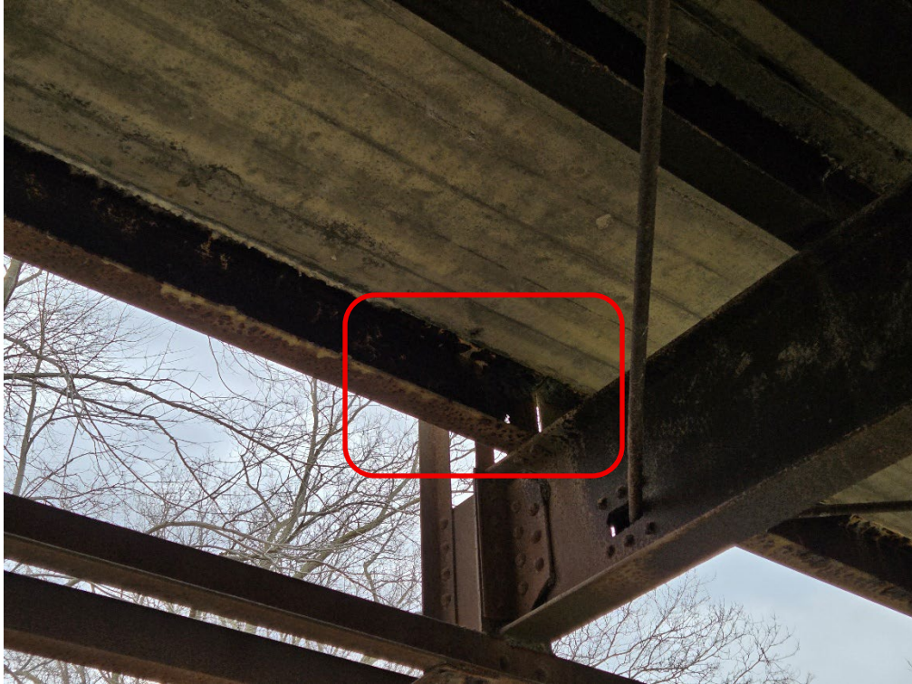
Perforation Through Stringer at SW Corner Above Transverse Beam
