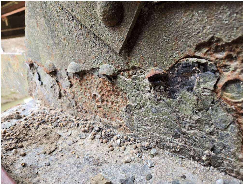
Typical Deterioration of Gussets and Rivets (East Side Interior Gusset at Midspan Shown)
